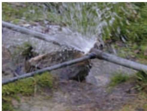
East Timor. Illegal Connections.
